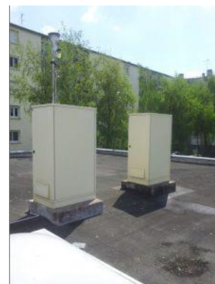
Figure 83 : Cabines de la station St Brieuc Balzac
